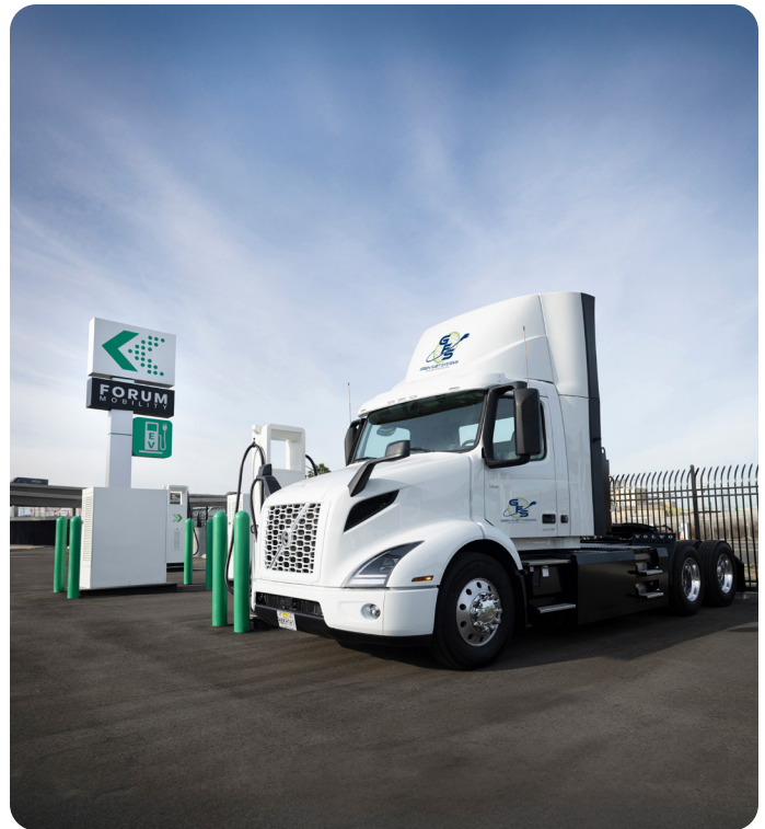
GFS Trucks charging at Forum Mobility's FM Harbor in Long Beach, CA, which offers 9MW of power at 44 charging dispensers.
